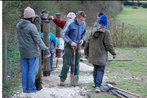
The first posts (cut from redundant telegraph poles) are dropped into place and firmly tamped-in.
