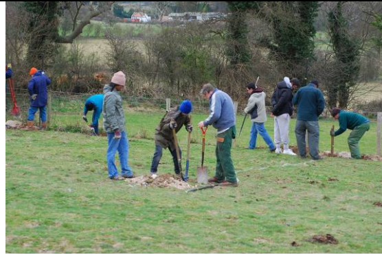
Site marked out and digging of 38 post-holes begins – each one metre down through hard chalk!
